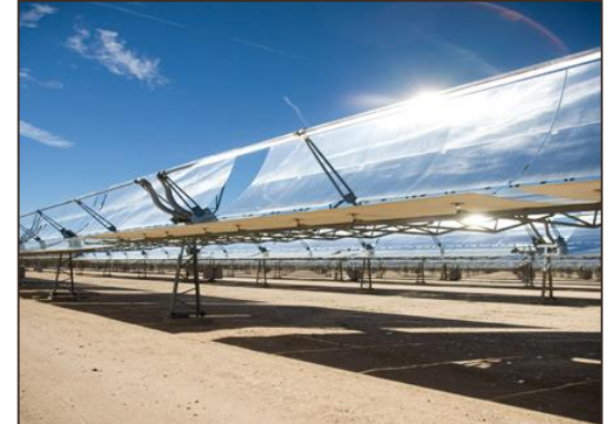
Concentrated Solar Power
